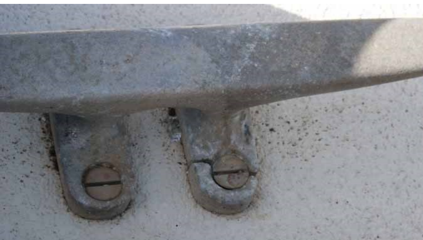
Stainless Steel Cleat Showing Corrosion Cracking
